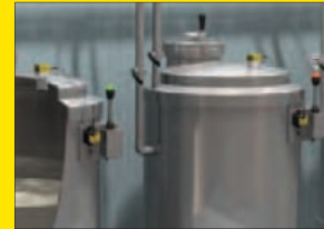
Tank Level Monitoring Status Indication K50L audible lights visibly and audibly alert operators when tank is filled to a certain point to prevent overflow.
