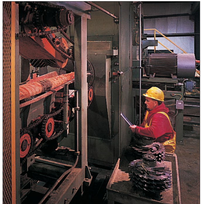
A Baldor•Reliance 500 Hp, medium voltage Severe Duty Motor (pictured at the back end of the machine) and Series 22H Line Regen Vector Control run this chipping machine at a North Carolina lumber mill. High performance and reliability are the hallmarks of this Baldor motor, running in multiple shifts, under high-torque demands, exposed to sawdust and other airborne contaminants.
